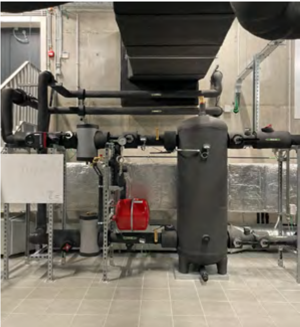
Kortrijk Weide, a DHC project in Belgium ©Agata Smok
