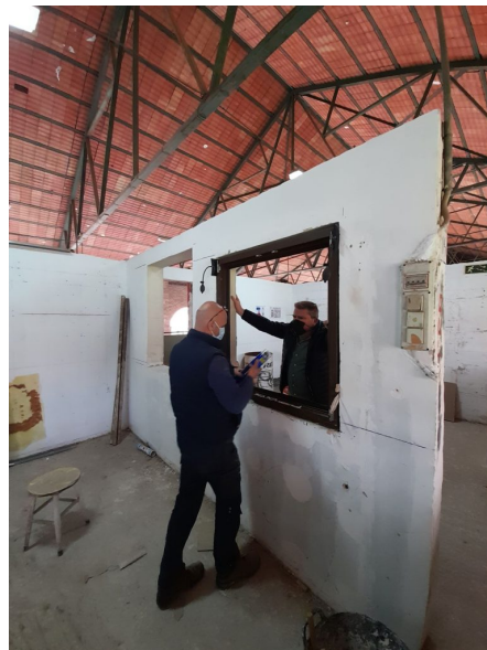
On-site assessment of energy efficiency skills of workers in Spain - © BUS League project
